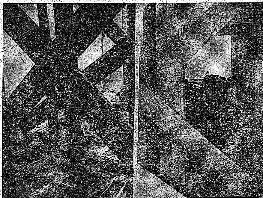
A view of the destroyed flat.
