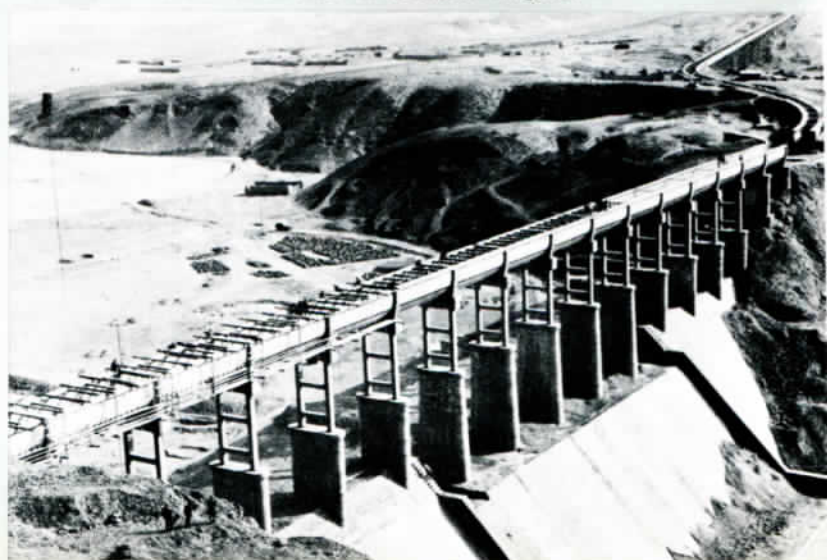
A large irrigation works on the Huanghe River is under construction in southern Ningxia.
