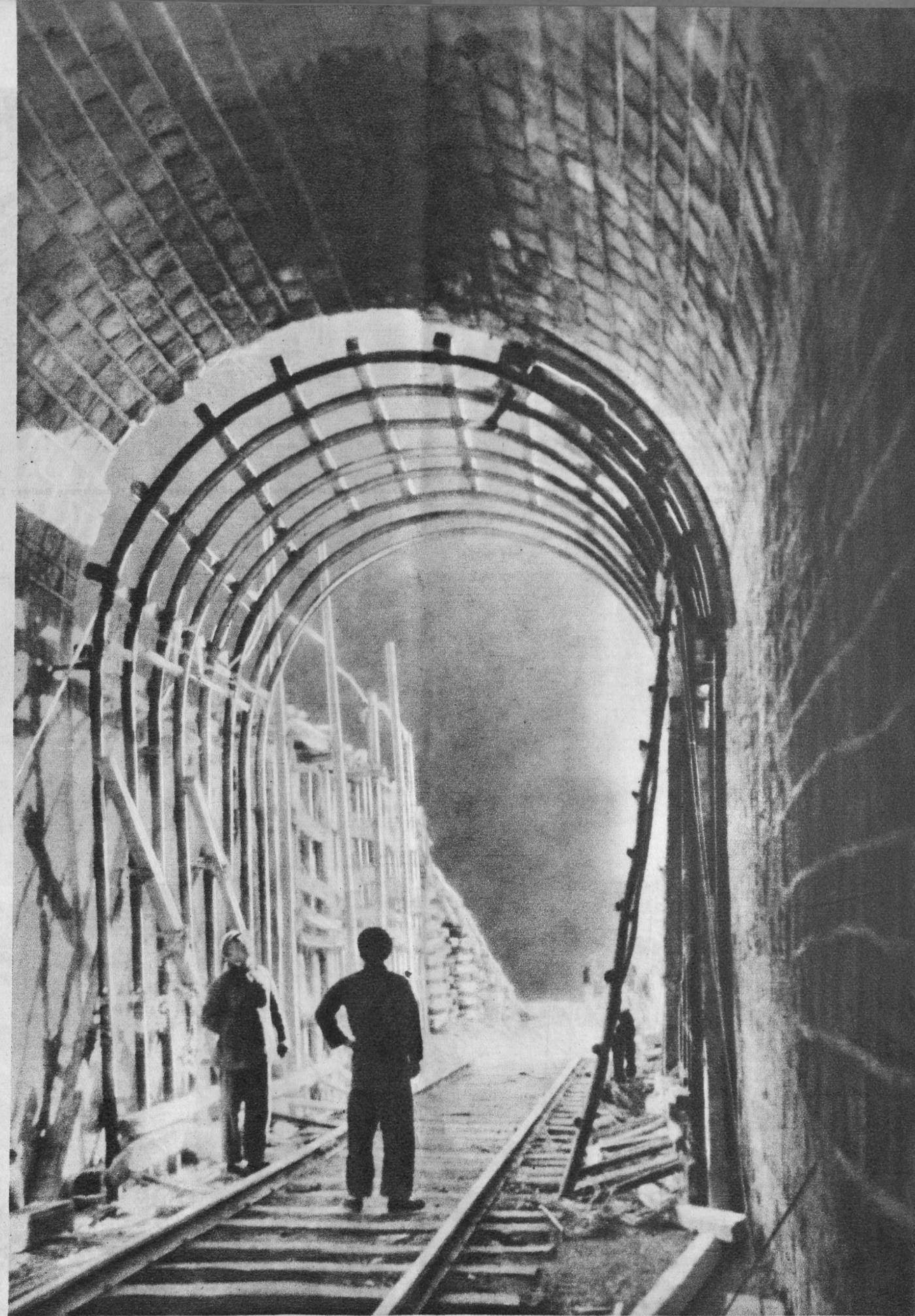
One of the many tunnels in construction on the Tienhui-Kanku Section of the line
