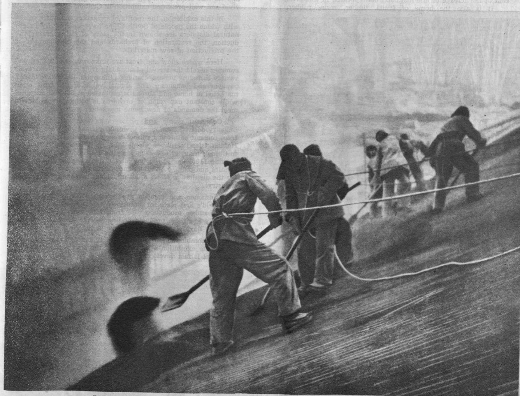
Dust has been removed from all parts of the buildings. Even the roofs came in for a spring-cleaning
