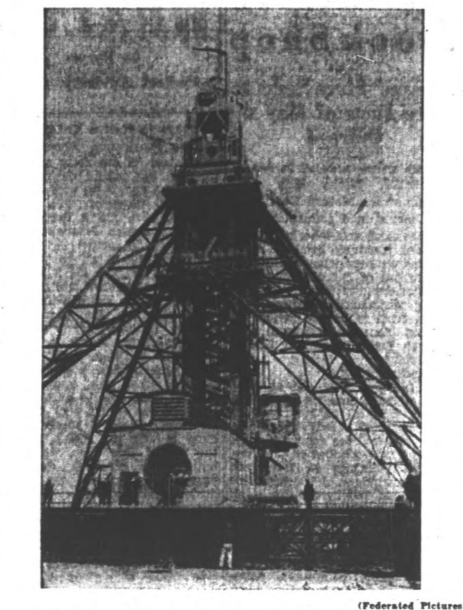
WPA workers at the naval station at Lakehurst, N. J., worked on this new mooring mast for the dirigible Von Hindenburg in its maiden flight from Germany to the United States.
