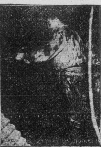
Digging away, 100 feet underground, this worker is helping to construct the first subway of the Soviet Union in Moscow. It is to be finished next year to help with the growing city's transportation problem.
