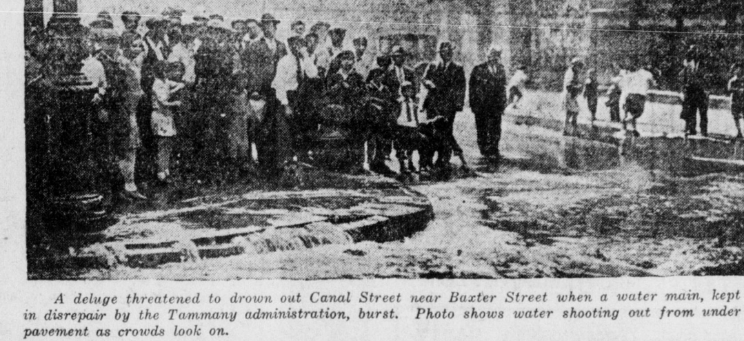
A deluge threatened to drown out Canal Street near Baxter Street when a water main, kept in disrepair by the Tammany administration, burst. Photo shows water shooting out from under pavement as crowds look on.
