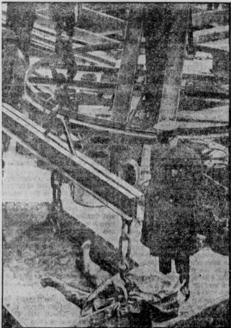
One worker was killed and seven injured in a dynamite blast in the ninety-foot pit in the new subway at 53rd street and 2nd avenue. Frank Harris, 38, colored, shown above, being carried to the shaft head, was killed in the explosion which trapped fifty workers.
