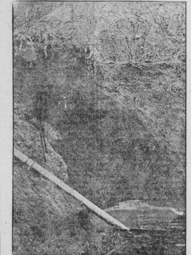
Using dynamite, rescuers try to reach ten men entombed in Claremont a cofferdam. The men were trapped seventy-five feet below the surface. Photo shows a wall of earth scores of feet thick separating the rescuers from the bodies. On the left is portal closed by the flood.
