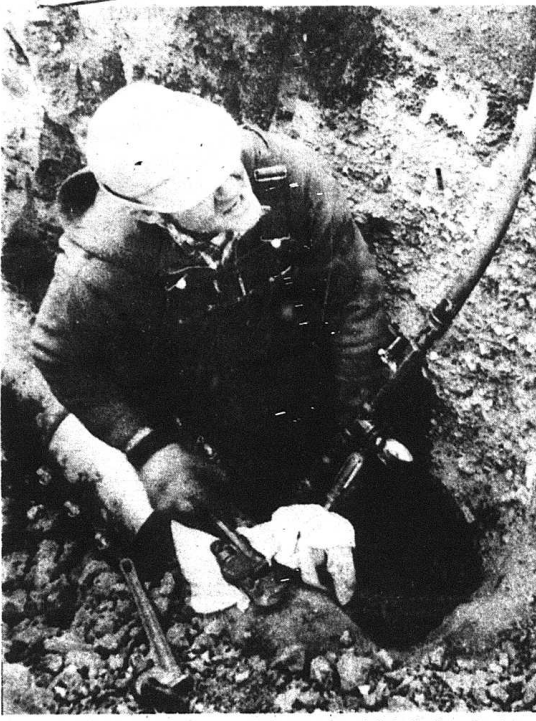
Working on gas pipeline: While gas companies claim pipeline shortages, the manufacturers are laying off workers because no orders are coming in.
