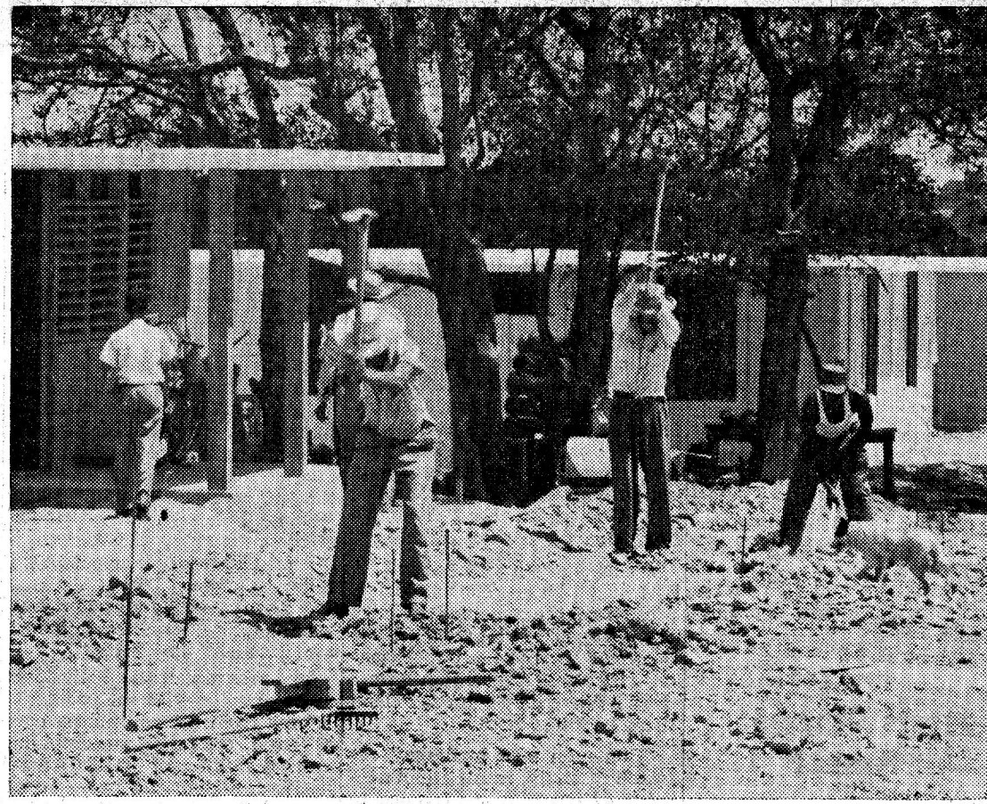
The old "bohio" with its palm-thatched roof and dirt floor is listed to go in Cuba. It will be replaced by model homes like these under construction — complete with inside plumbing. Members of the co-operatives don't mind the hard work or the primitive tools because they're building their own homes with government help. The perspective of a new Cuba, completely modernized, was made possible by the revolution that overthrew the Batista dictatorship.
