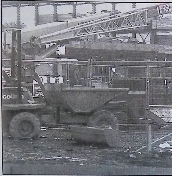
Builders marched onto a Collen site in East Wall and took this photo. Note the lack of safety rail and inadequate scaffolding. This is potentially lethal.
