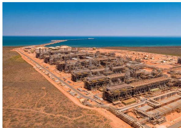
Gorgon LNG plant in Western Australia – owned by US multinational Chevron
